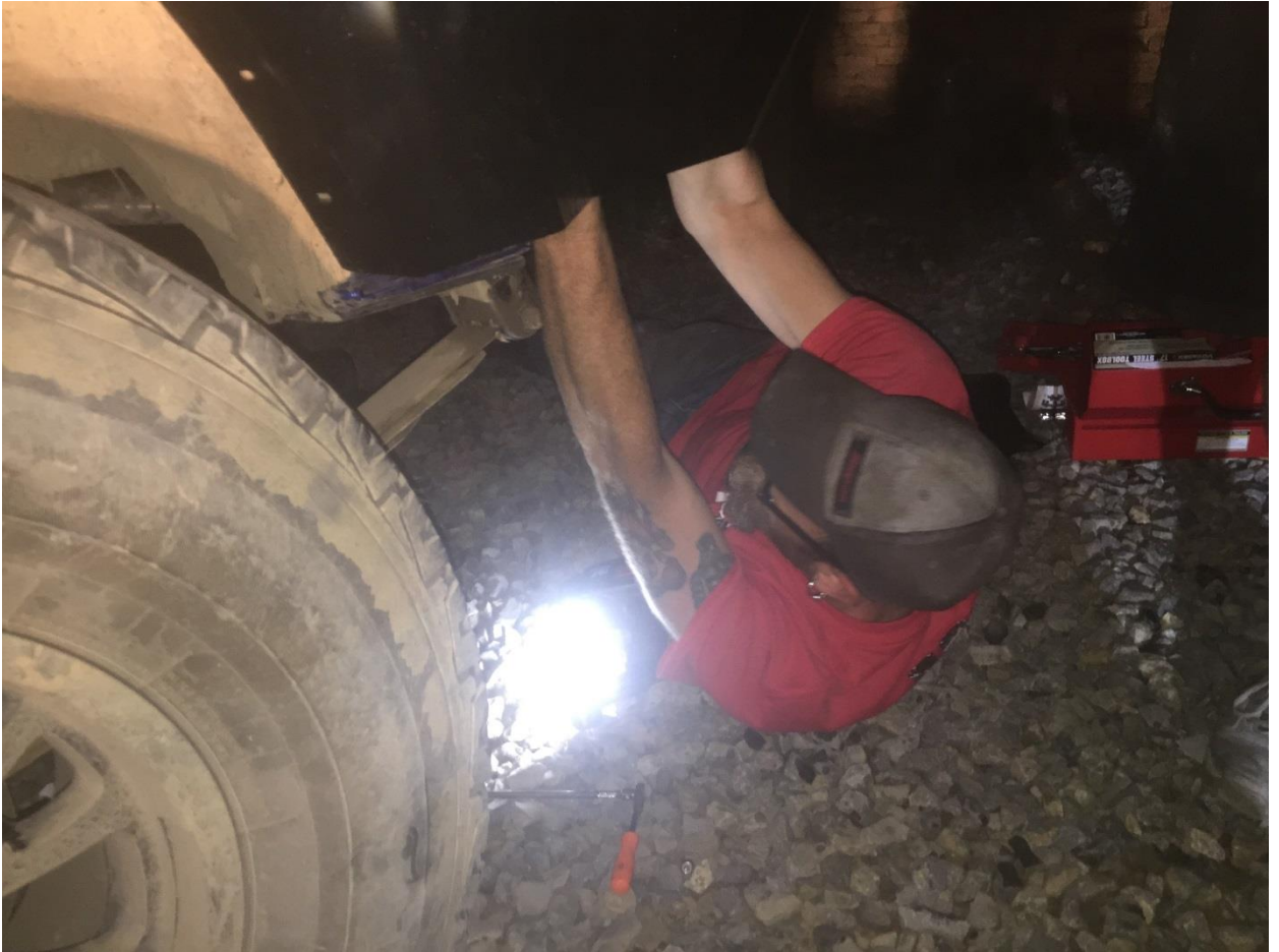
Figure 3e - When reaching in from the bottom to insert the carriage bolts in the top bracket or start the nuts on the carriage bolts, it helps to have Rob Lowe arms.
