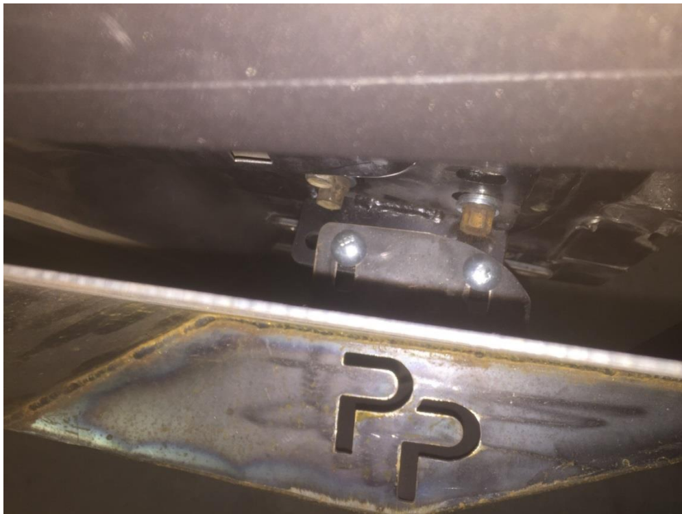
Figure 3b, 3c, & 3d – Bolts placed through corner bracket and main support bracket
